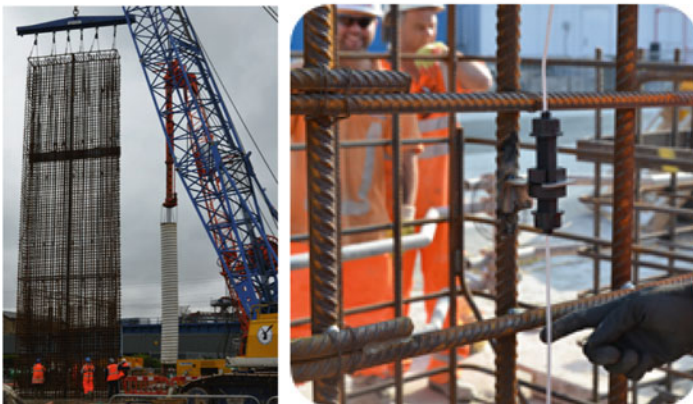
Fig. 21.4 Examples of FO strain measurement in geotechnical structures by Cambridge University and CSIC. (a) Piles. (b) Tunnels. (c) Diaphragm walls
