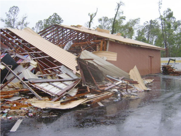
Fig. 14.8 Collapse of a wood-frame (metal clad) building
