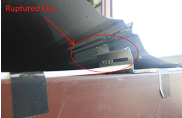
Fig. 17.15 Clip rupture at the free high-eave corner (Chowdhury et al. 2014)
