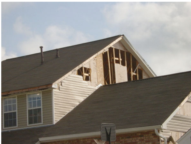
Fig. 14.6 Gable-end damage during Hurricane Katrina
