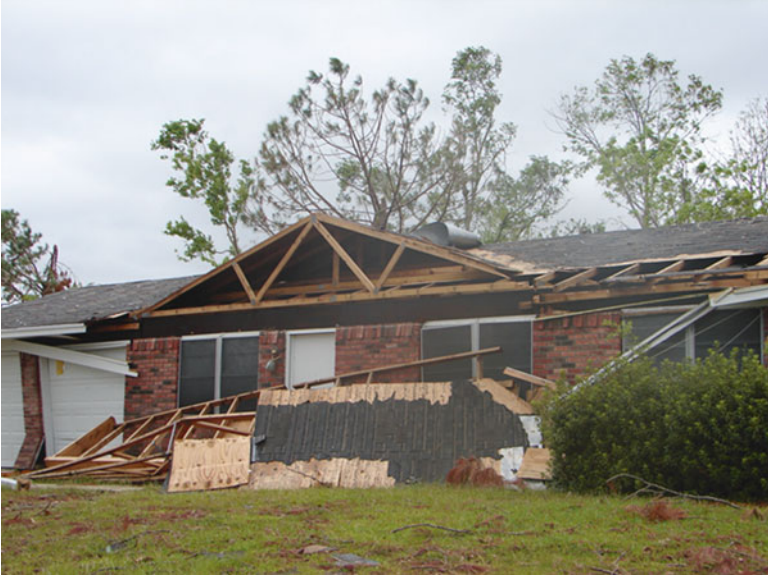
Fig. 14.7 Loss of a porch overhang due to lack of support post anchorage
