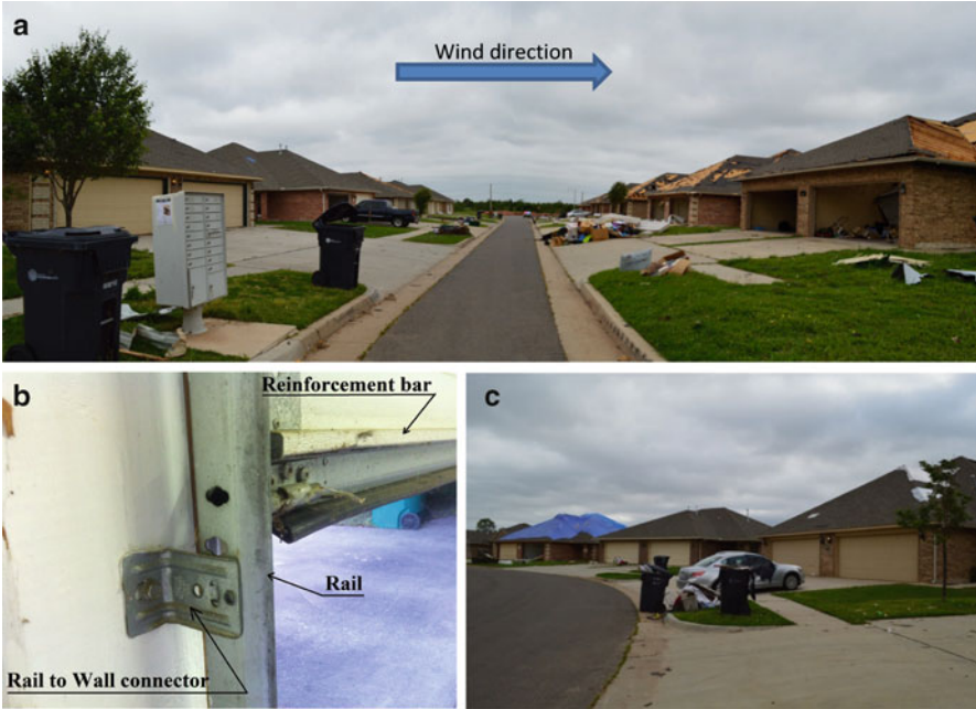
Fig. 14.3 Different garage door damage levels on the same street. (a) Leeward (left) and windward (right) sides of SW 151st Street. (b) Garage door supports and configuration. (c) Change of garage door damage level when home orientation changes from leeward to windward direction
